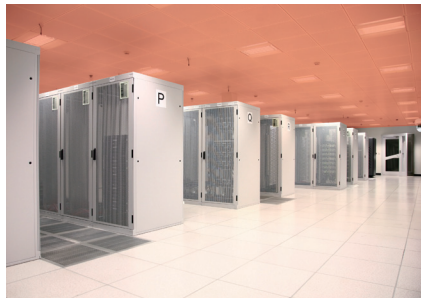
Ceiling protection at Data center
